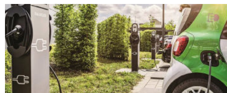
EV Charging Station. Photo Courtesy of PV Magazine
